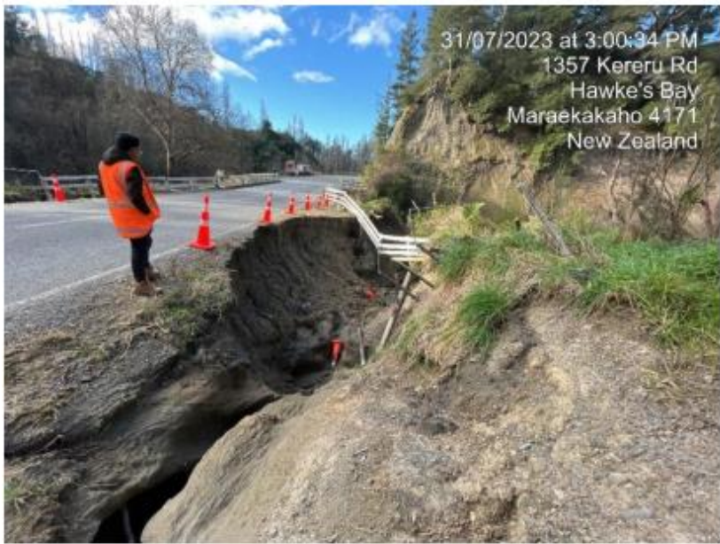
Figure 3-2: Site photo of eastbound road shoulder slip at Kereru Road RP12.808 facing north remedial works)
