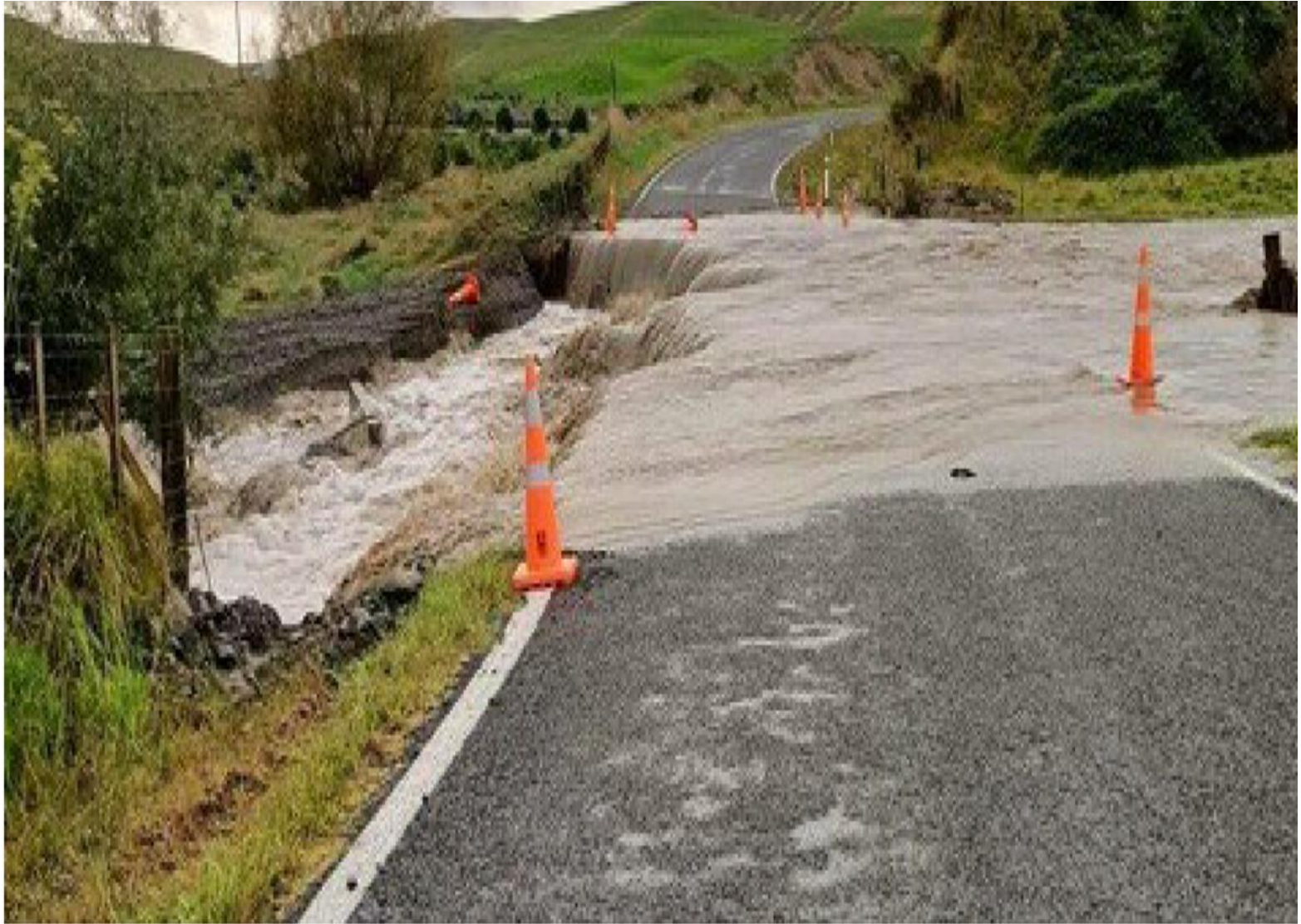
Figure 2 Salisbury Rd overtopped on 14 th March 2023
