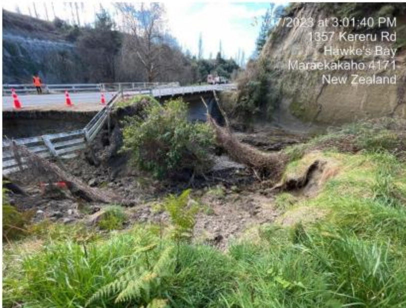
Figure 3-3: Site photo of eastbound road shoulder slip at Kereru Road RP12.808 facing north remedial works)
